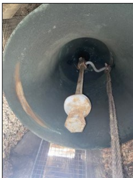
Wear mark on bell
